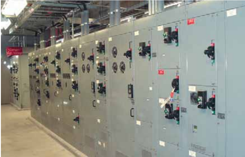
ControlLogix PACs manage all of the MCCs deployed throughout the sugar mill. DeviceNet connects the MCC starters to the PACs. For each MCC, just one DeviceNet cable replaces hundreds of control wires, making installation and maintenance much easier.
